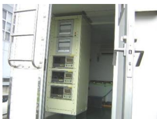
Automatic air quality measurement device
